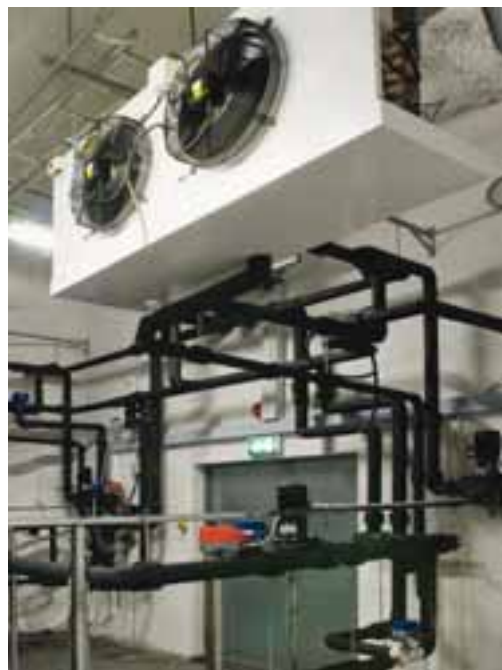
Kuldeanlegg / Refrigeration plant
